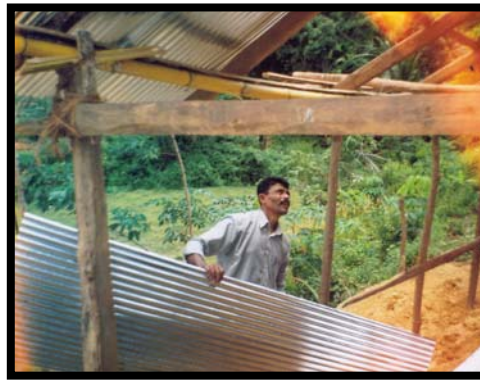
Aug 24 th : Our "spare change" put the roof on the woman's new home.
